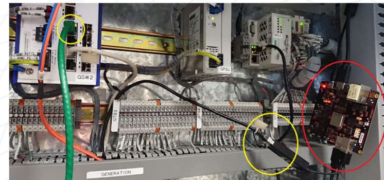
BITW device integrated into EPIC Testbed
